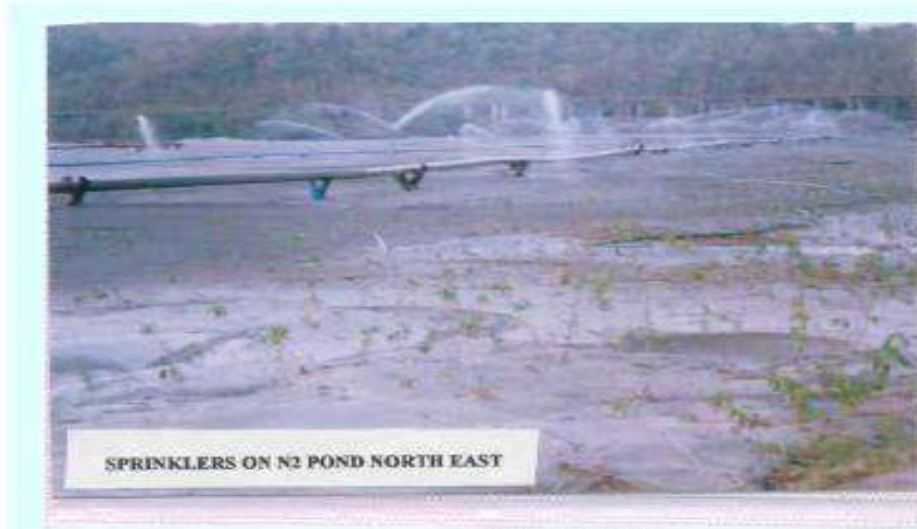
a) Safe Disposal for Control of Fugitive Dust with Sprinkler
